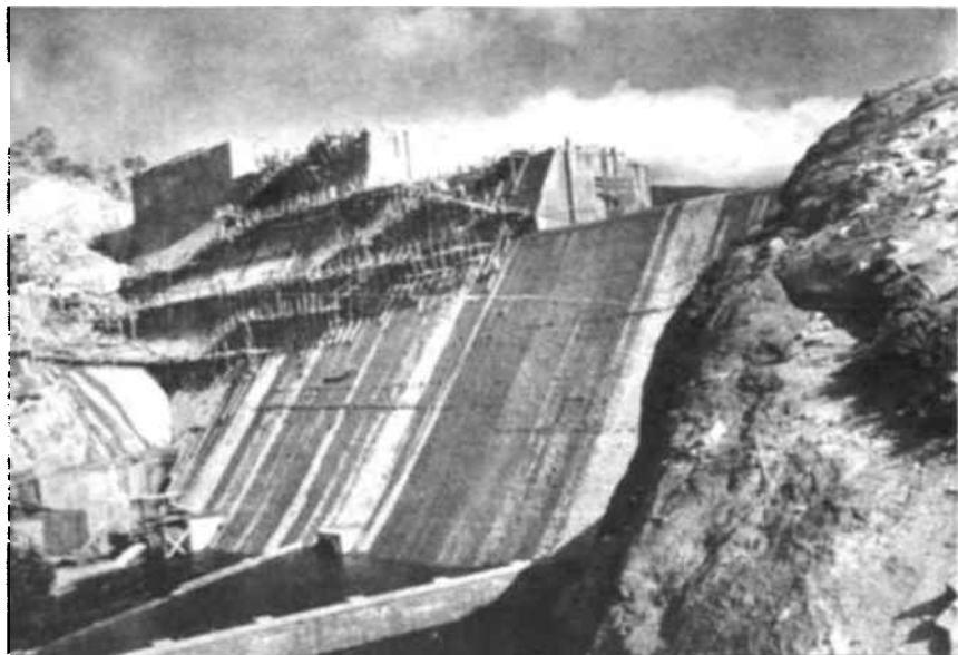
One of the many dams under construction in India today—part of the vast schemes undertaken by the Government to harness natural resources in order to raise India out of poverty, and provide her people with a higher standard of living.
